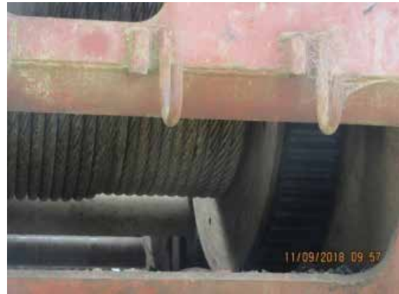
Guard missing over exposed gearing and moving ropes
