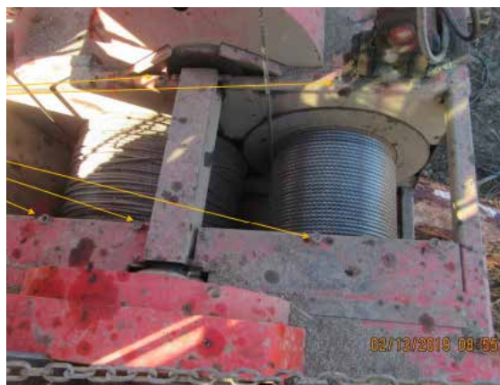
OEM handrails missing on a swing yarder winch set – original mounting points arrowed.
