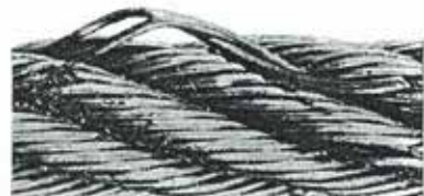
10. Wire fractures at the strand, or core interfaces, as distinct from 'crowns' fractures, caused by failure of core support.
