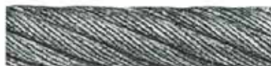
7. Corrosion of severe degree caused by immersion of rope in chemically treated water.
