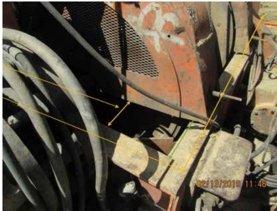
Incomplete guard over clutch adjacent to (substandard) walkway used to access far side of machine.
