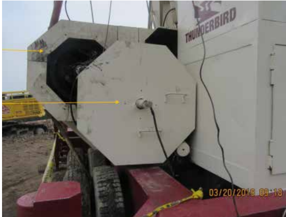
Guards removed and not replaced. Bolt holes visible where arrowed.
