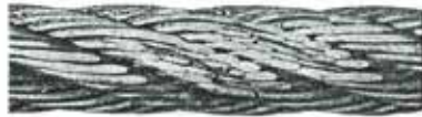
2. Localised wear due to abrasion on supporting structure. Vibration of rope between drum and jib head sheave.
