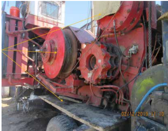
Unguarded rotating machinery accessed by unsafe walkway - lack of: sufficient clearances, handrails/kickplates, non-slip walkway surface.
