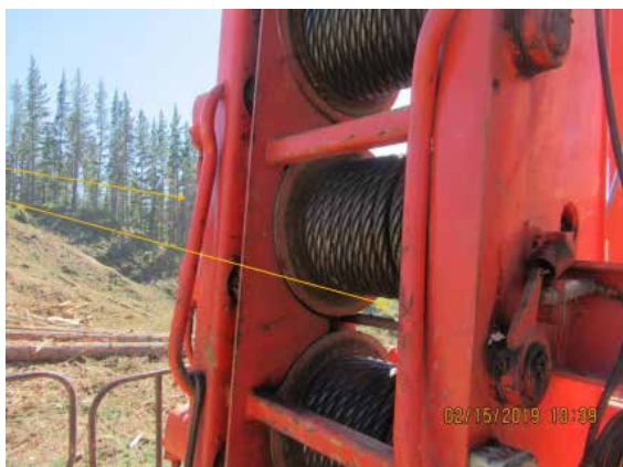
Worker access to gantry ladder is by climbing up guy winches (less than ideal) and where the handrails have been crushed (dangerous).
