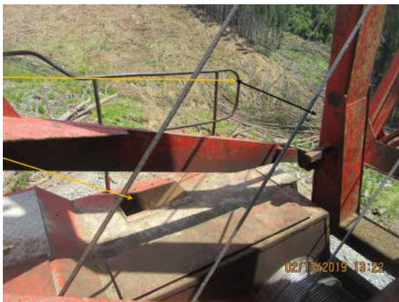
Similarly, handrail open at ends and no kick plates.
